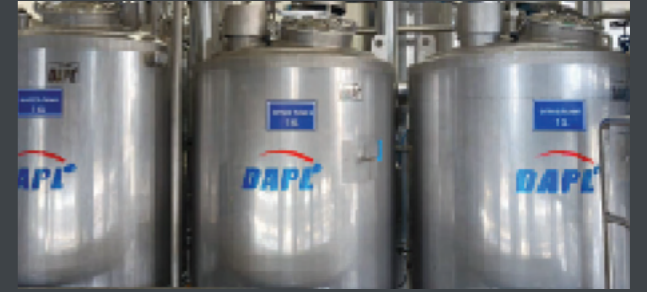
MILK STORAGE TANK
